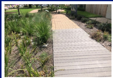
Rain garden with a permeable footpath located in Bayou Metairie Park; credit: Richard Gillen
