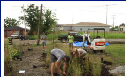
Rain Garden Installation in Hollygrove completed by the Small Center at Tulane University, in partnership with the Carrollton Hollygrove Community Development Corporation; source: small.tulane.edu
